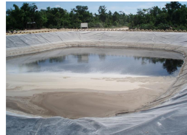
Lined Evaporation pond
