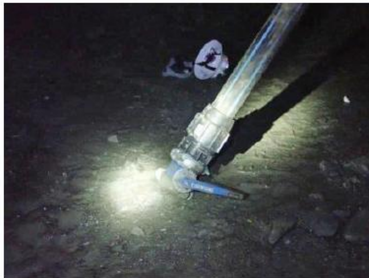
View of the failed coupling.
