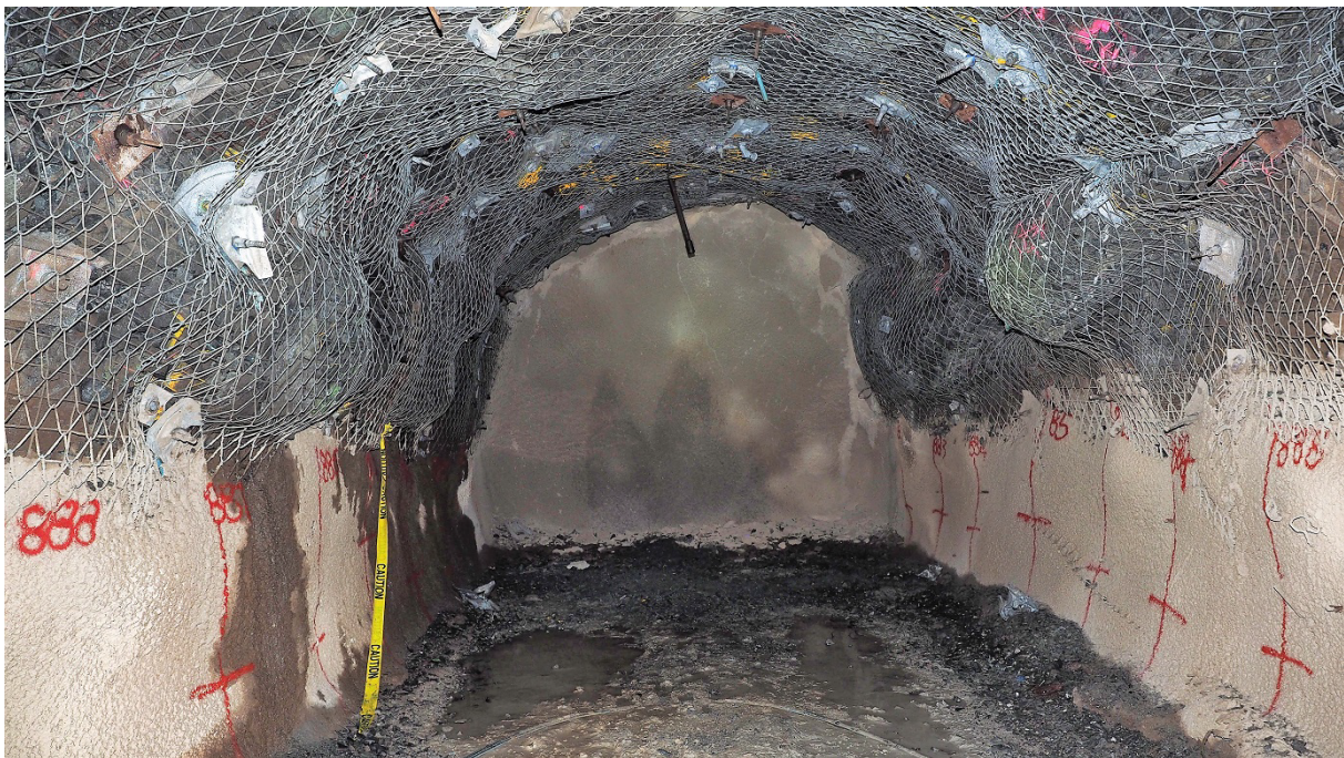
FIG 10 – Performance of a single-layered high energy dissipation ground support scheme following a +1.9 ML seismic event and associated dynamic loading. Rehabilitation was not required due to the remaining load-bearing capacity.
