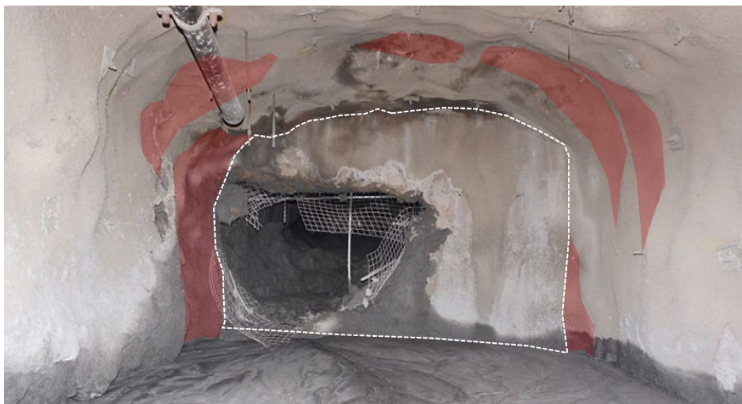
FIG 10 – Consideration of a negative abutment angle at the location of the barricade failure.
