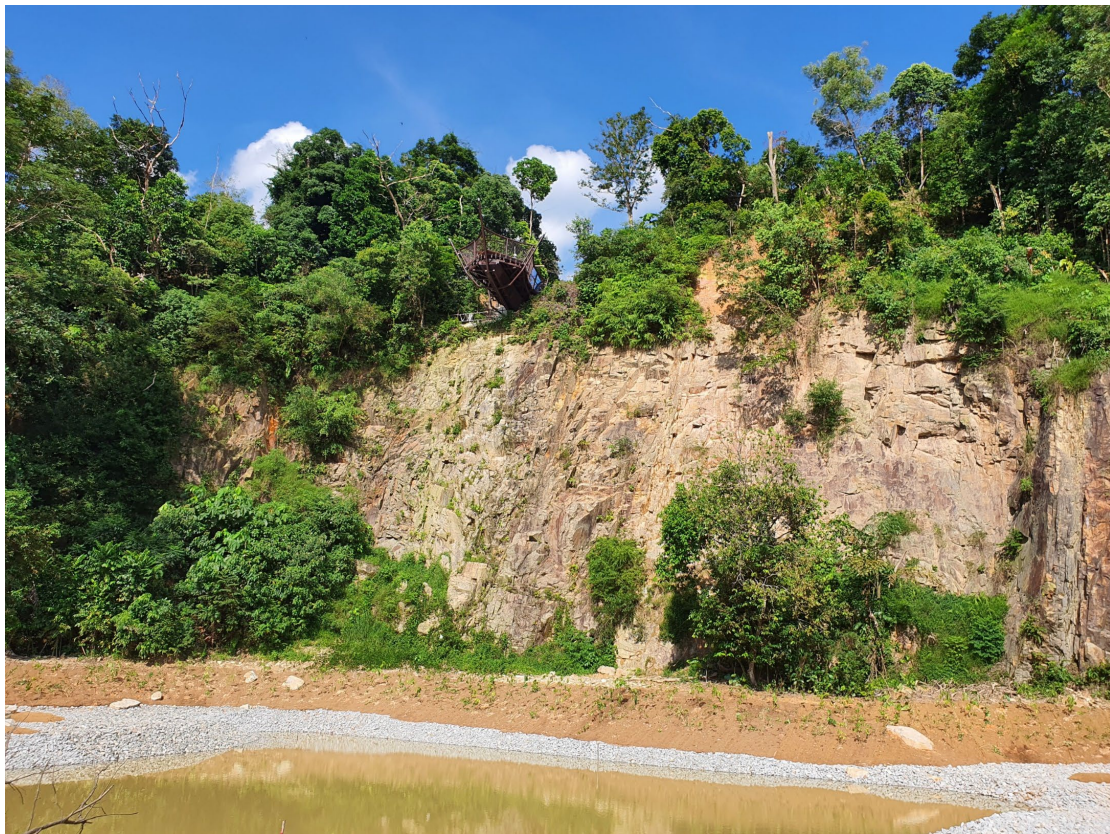
FIG 9 – Overall rock slope condition after scaling work with colugo deck structure on top.
