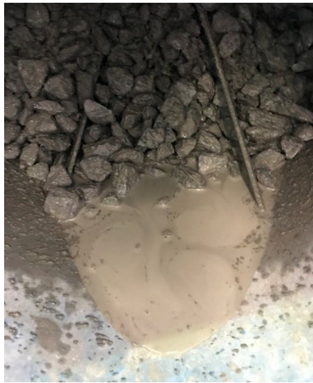
FIG 7 – CRF mix in concrete mixer showing segregation. Note the slurry is too runny and is not coating and clinging to the aggregates.
