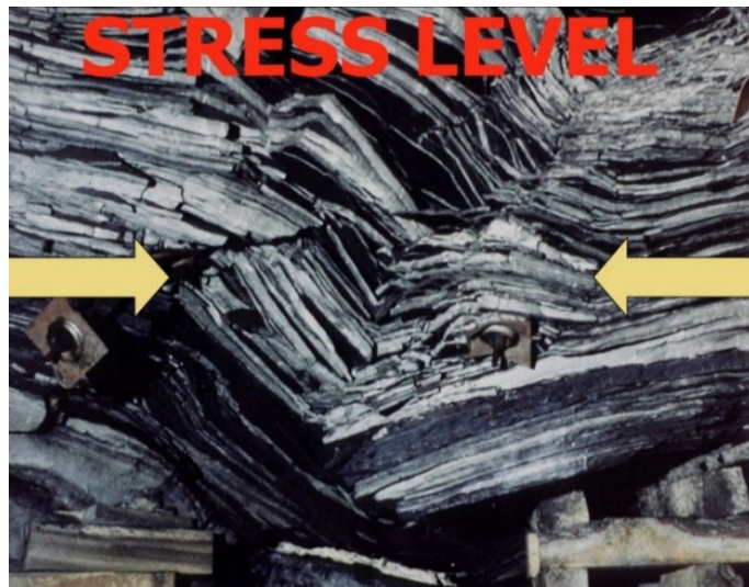
FIG 7 – Coalmine roadway roof displaying buckling and shear/tensile failure due to horizontal stress.
