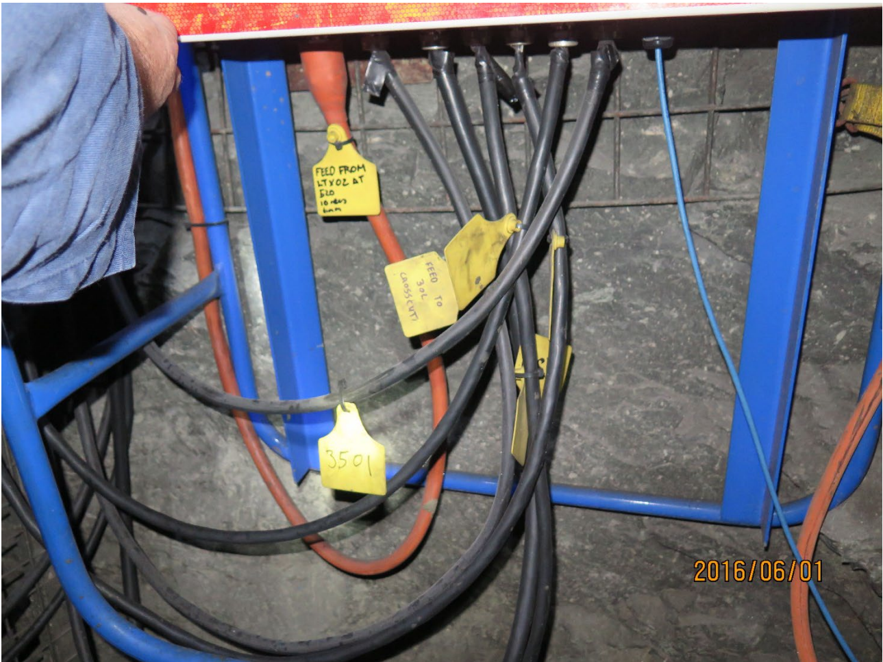
FIG 11 – Well labelled cables but poorly terminated into the enclosure.
