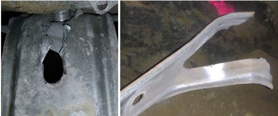
FIG 14 – Tearing around securing bolts; left – sample 4 round hole that has become elongate as the strap pulled a considerable distance past the securing bolt; right – sample 7 elongate hole has torn through to the end of the strap disconnecting it from the securing bolt.
