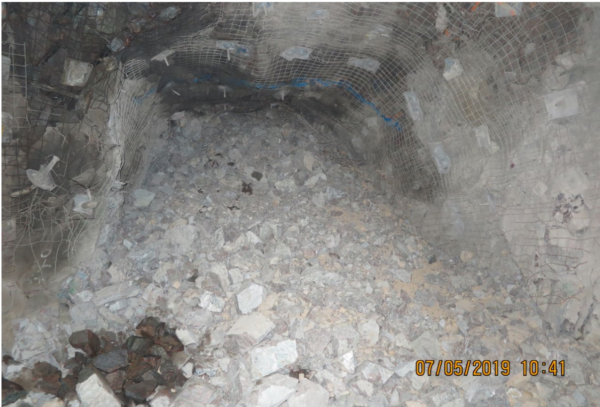
FIG 6 – ‘Light’ ground support at a SLC brow region, consisting of resin bolts and weld mesh.
