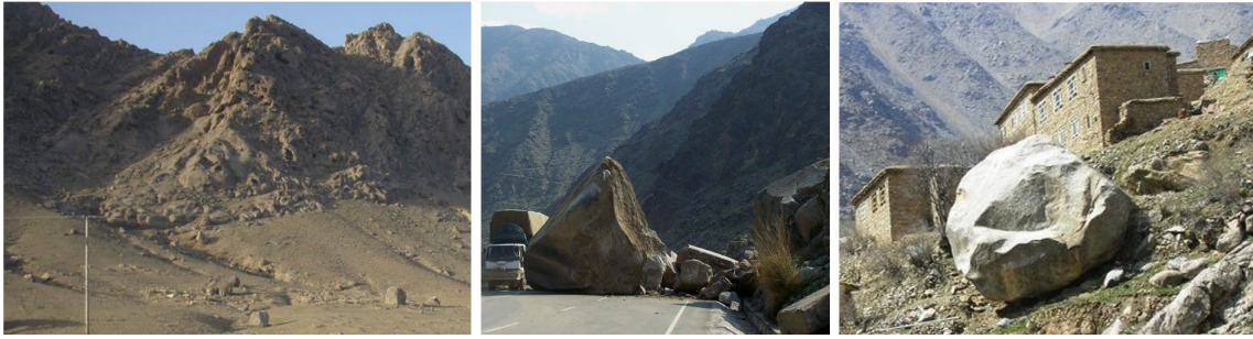
FIG 7 – Slope failures belonging to Category III involving rockfalls.
