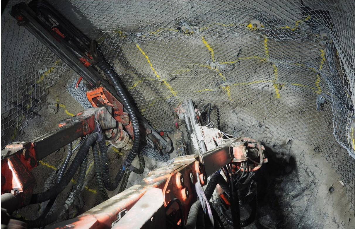
FIG 11 – Installation of high-tensile chain-link mesh surface support in deep mine development using a conventional twin-boom jumbo (Goldfields region, Western Australia).
