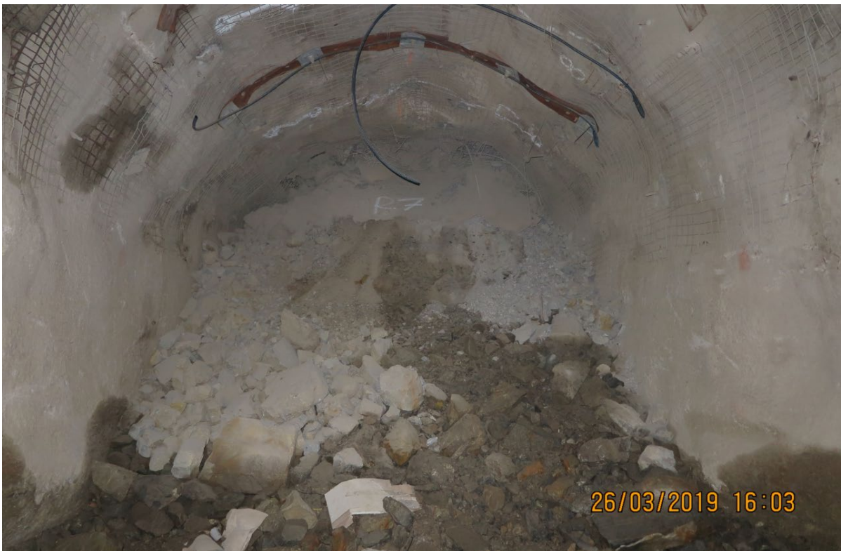
FIG 7 – ‘Heavy’ ground support at a SLC brow region, consisting of fibrecrete to floor, weld mesh to 3.5 m from the floor with resin bolts, and a second pass of ground support including W straps and hybrid bolts.
