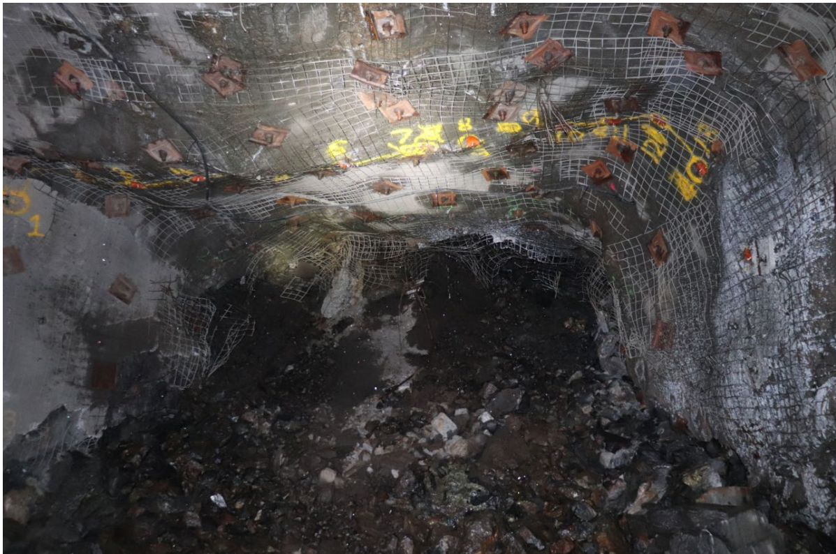
FIG 8 – ‘Very heavy’ ground support at a SLC brow region, consisting of fibrecrete to floor, weld mesh to 1 m from the floor installed with resin bolts, and a second pass of ground support including mesh straps, hybrid bolts and cablebolts.
