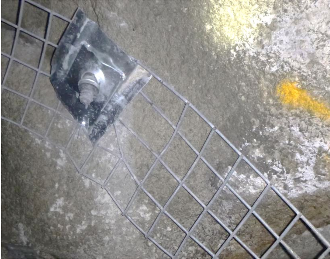
FIG 10 – Mesh strap centre sample 3 ‘LH’ securing bolt failed lateral wires.
