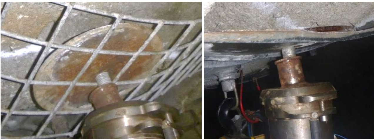
FIG 4 – Steel load transfer plate installed behind Mesh strap (left) and behind W-strap (right), also showing the top of the DTR coupling unit attached to the plate in readiness for a test.
