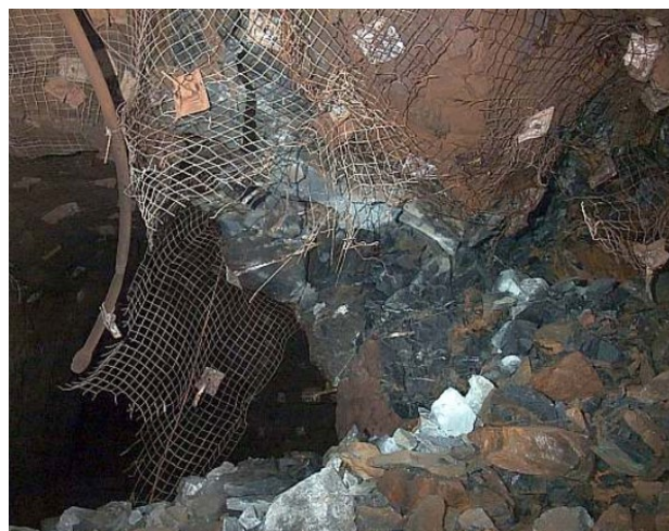
FIG 7 – Crush damage to pillar nose in the disused 1606, due to the ML 2.1 event immediately after the 15 Level TSB firing. Damage included two snapped Posimix bolts, torn mesh, and 80 t rock displaced.
