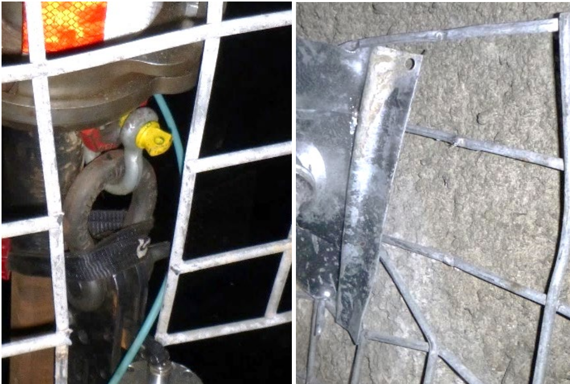
FIG 11 – Mesh cross strap failure mode – left: sample 1 rupture; right: sample 3 weld failure.
