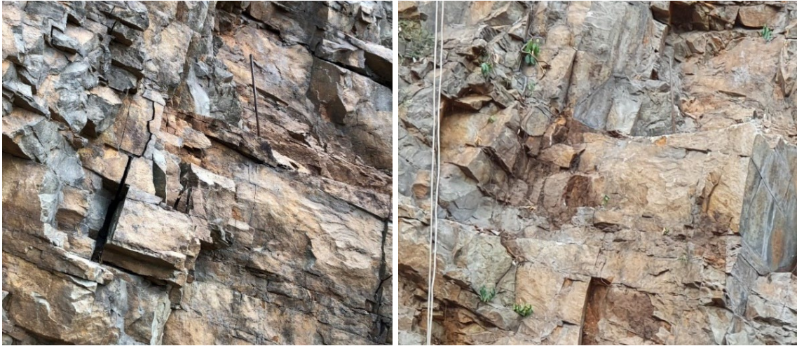
FIG 8 – Comparison of rock slope condition before scaling work (left photo) versus after scaling work (right photo) at some selected locations.
