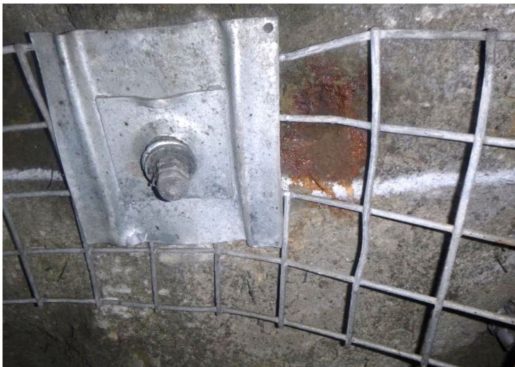
FIG 9 – Mesh strap end sample 2 – 'LH' securing bolt failed wires.
