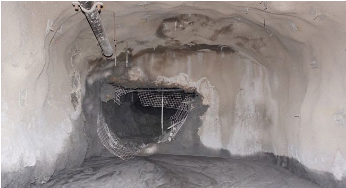
FIG 3 – Drive side of failed paste wall with fill pipe through wall (after Department of Mines, 2020).
