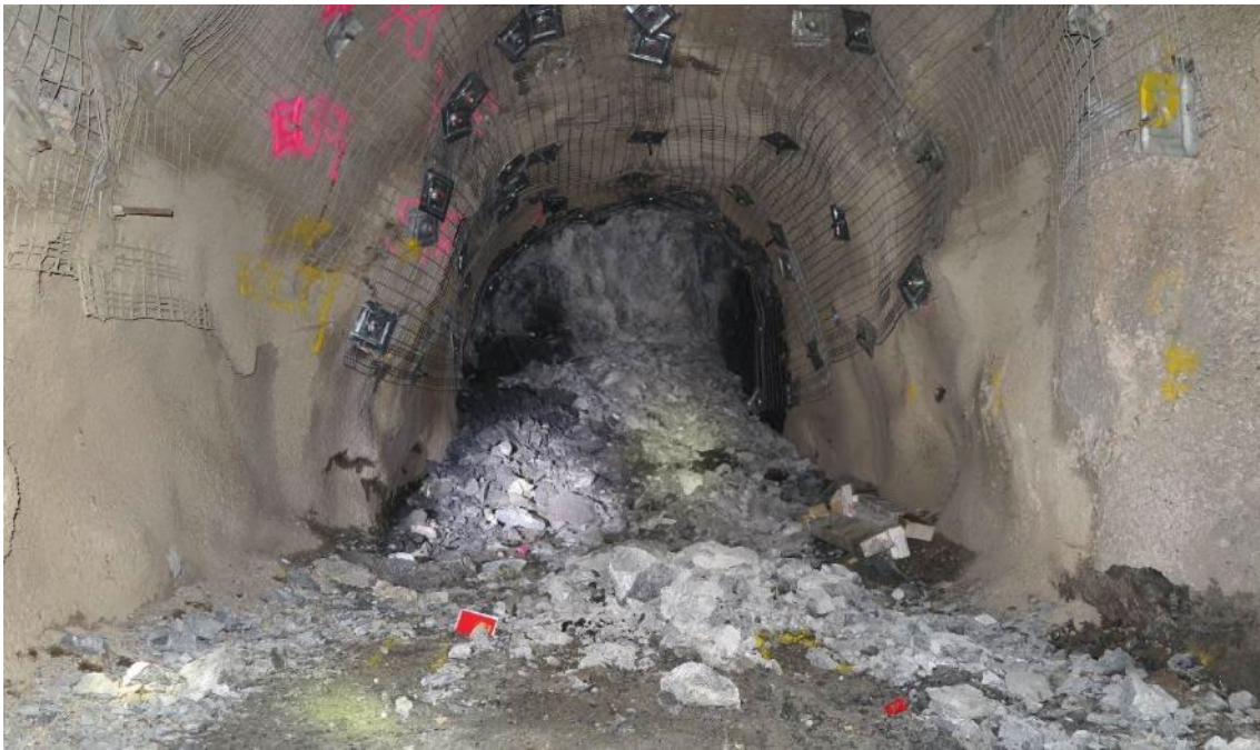
FIG 1 – Violent stress-driven instability of a development face with a significant ejection distance.
