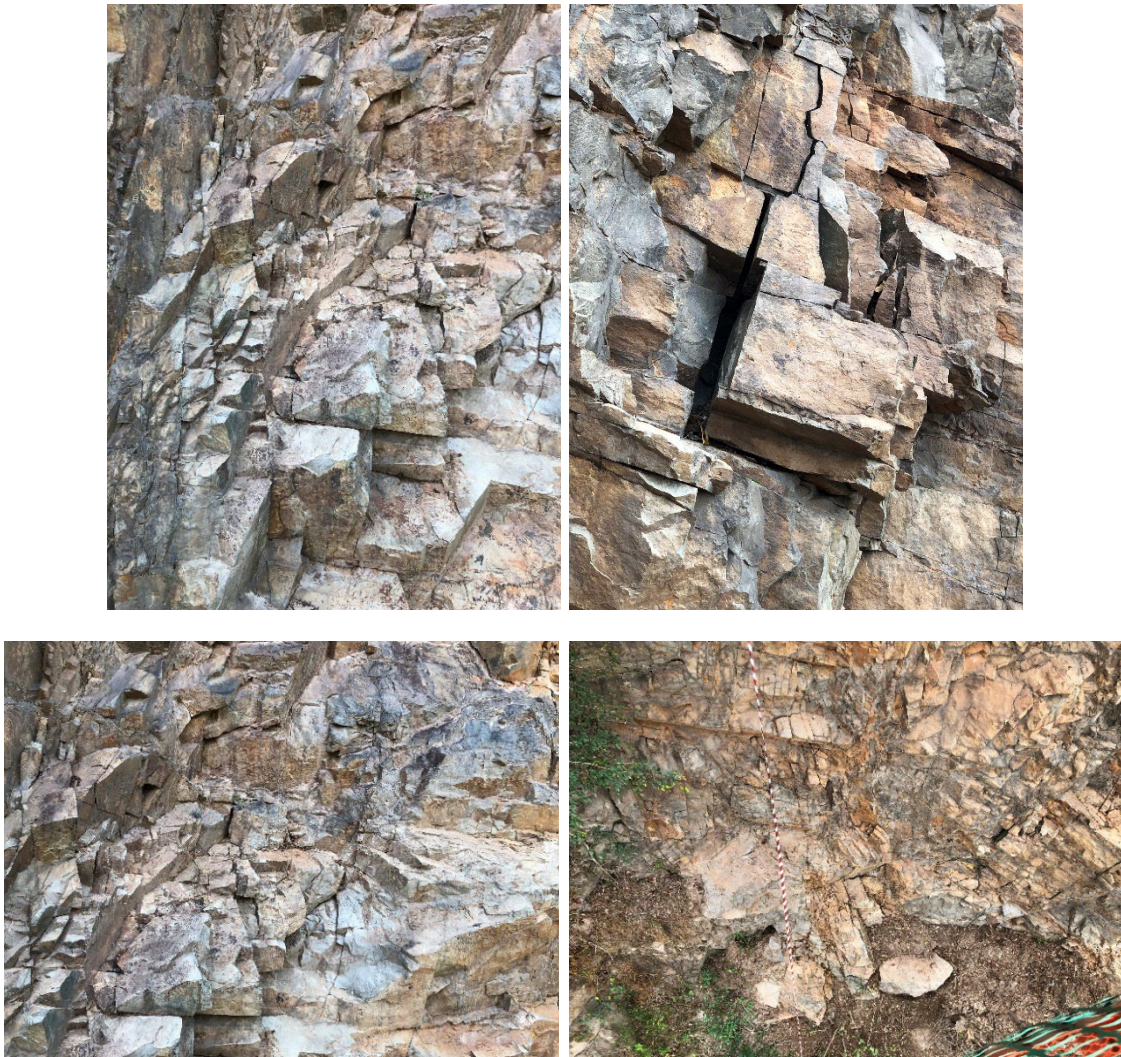
FIG 5 – Observed loosely attached rock pieces on different locations on rock slope (case 2 area).
