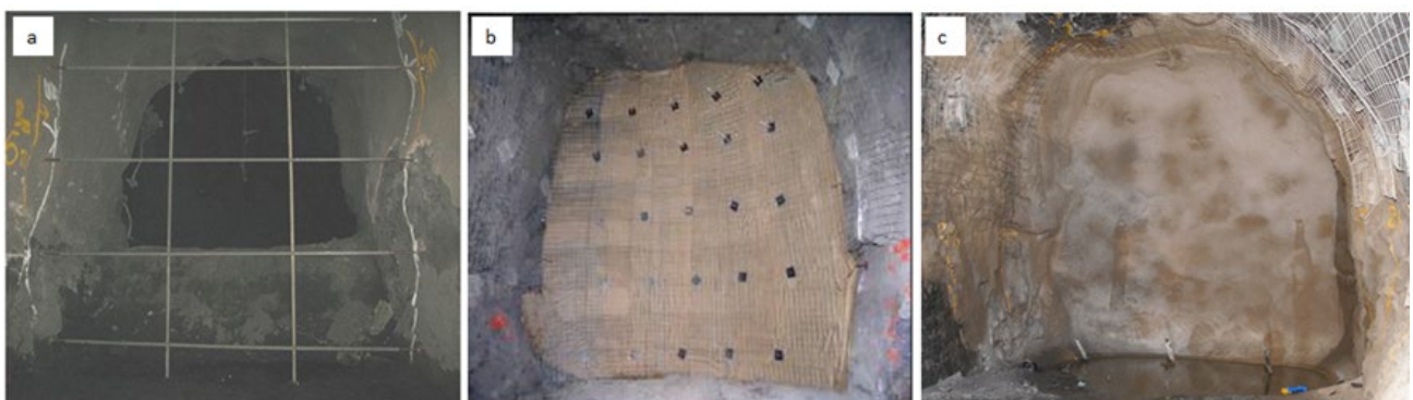
FIG 2 – Formwork and steps of construction of fibrecrete bulkheads (a) pre-fabricated arch placement (b) placement of the mesh and hessian over the arch (c) sprayed fibrecrete.
