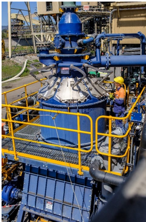
FIG 1 – Photograph of the skid-mounted single-stage separator installed on-site.
