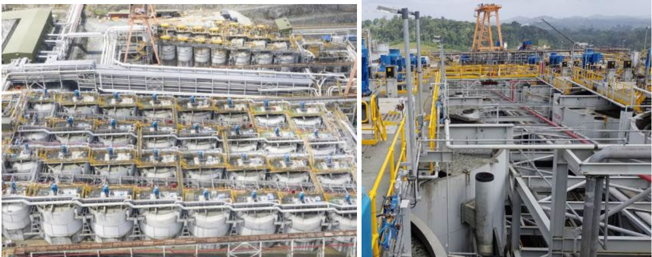
FIG 1 – Cobre Panama is the first large scale greenfield copper operation designed and built with TankCell® e630 technology.
