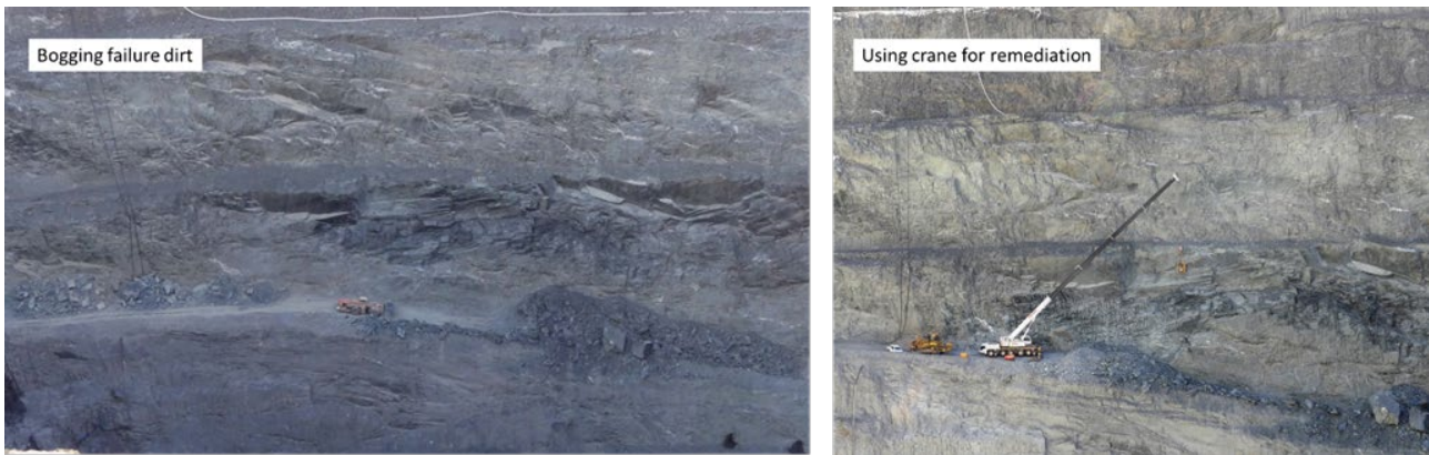
FIG 12 – Underground remote loader removing failed material and remediation using crane with man basket attachment.
