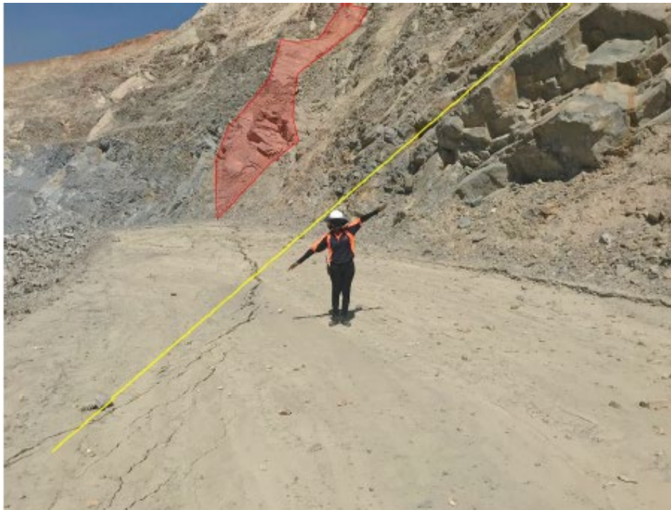
Figure 3-6 Pit 5A Access Ramp, location of distressed section. Orientation of J2 (yellow) demonstrated by Weatherly Geologist. J1 shown in red. Note tension cracks on access ramp prior to failure.
